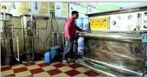
RO Water Plant
