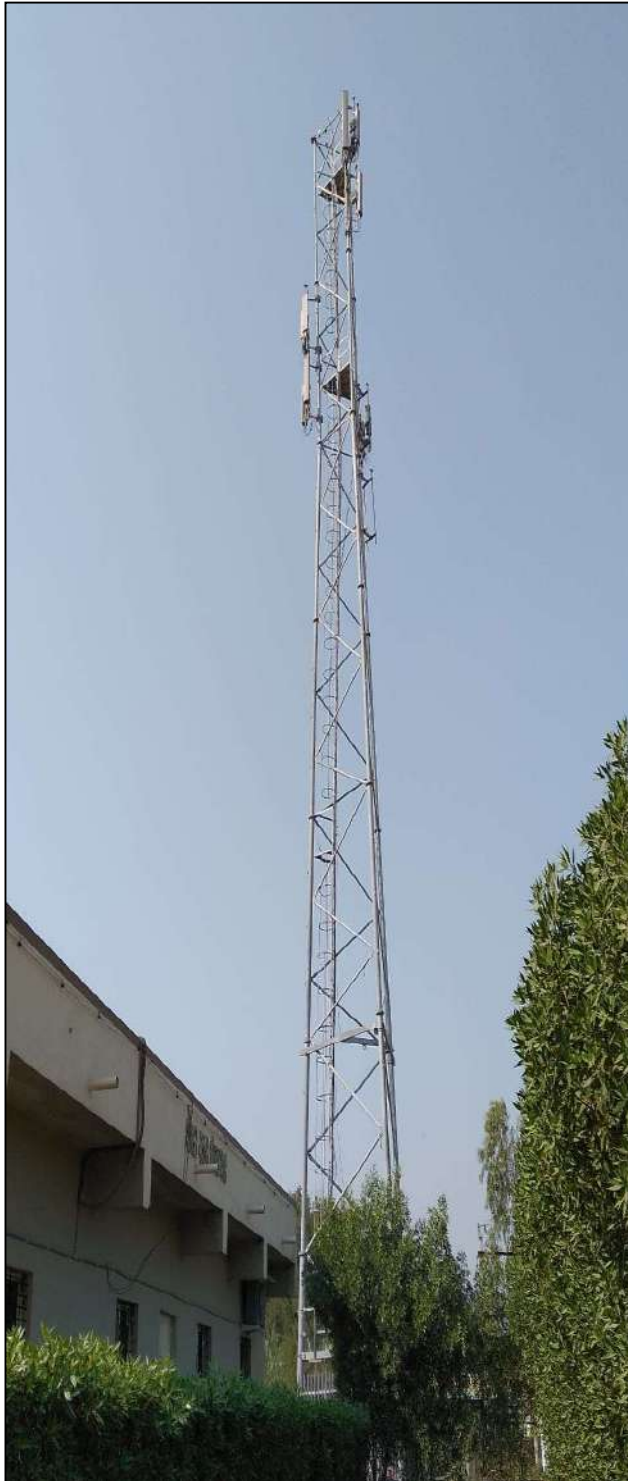
FIG.51: MOBILE NETWORK TOWER
