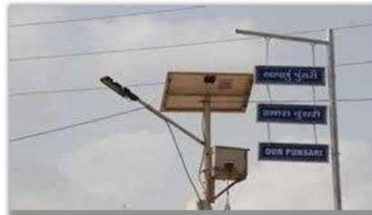
Solar Street Light
